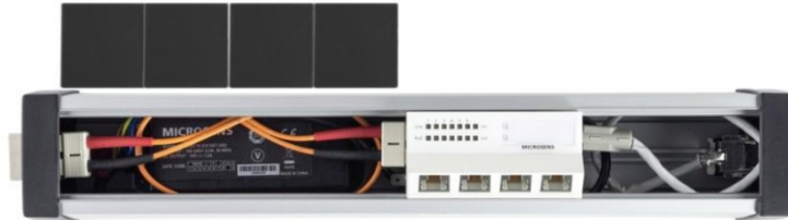
Micro Switch installed with a power supply in an MS140131GT-8
